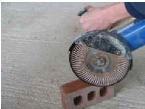
using an angle grinder for engineering bricks.... remember safety first when using power tools
